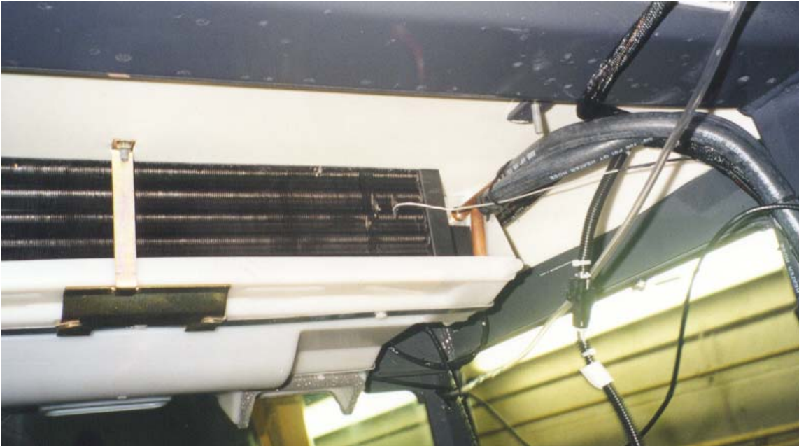
Heater tube end of evaporator coil.
